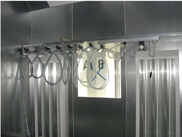
C-Rail system at the finishing area of a car production
