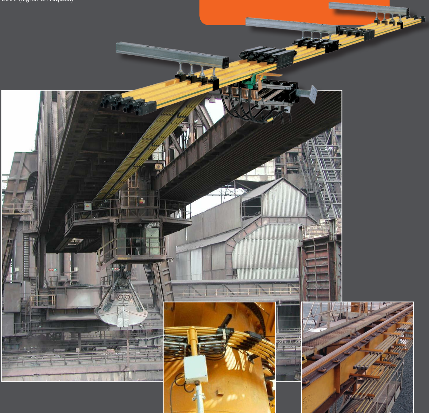
Conductor Rails on a boom stacker
